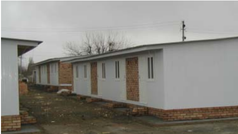
The 180 rooms constructed for Chechen displaced families by MSF, which have been declared illegal.
